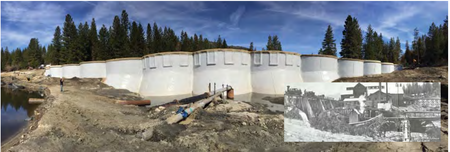
Hume Lake Dam after rehabilitation. Inset: Photo of the dam taken in the early 1900s when the lumber mills was in full operation.
