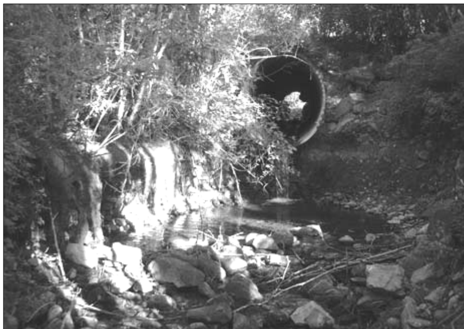
Bank undercutting at culvert outlet effectively preventing the passage of fish and other aquatic organisms.
