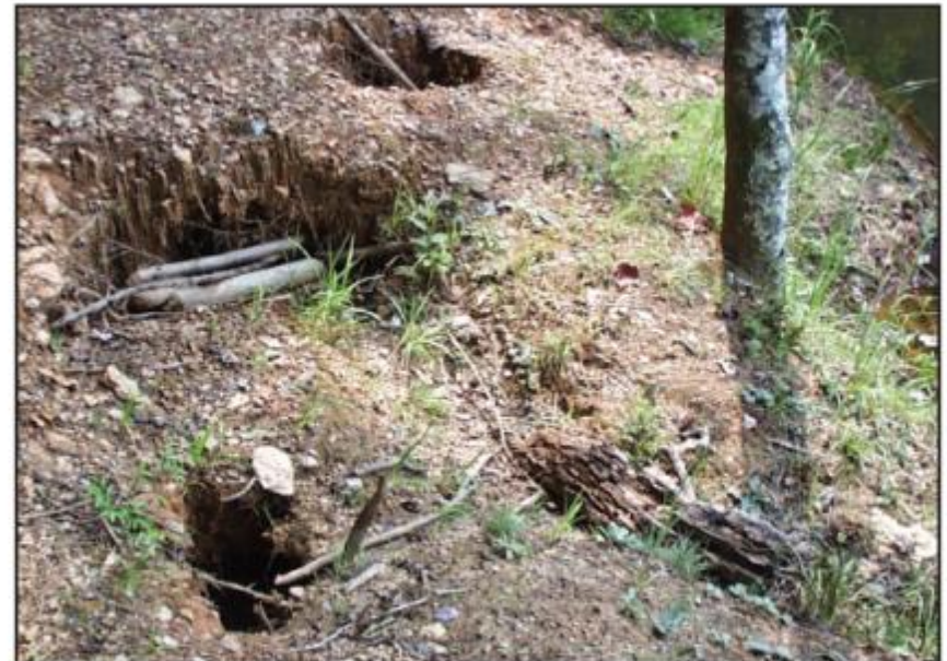
Figure 16—Rodent holes in the dam face can cause dam failure.
