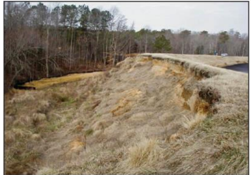
Figure 8—Slumping on the downstream face of a dam.
