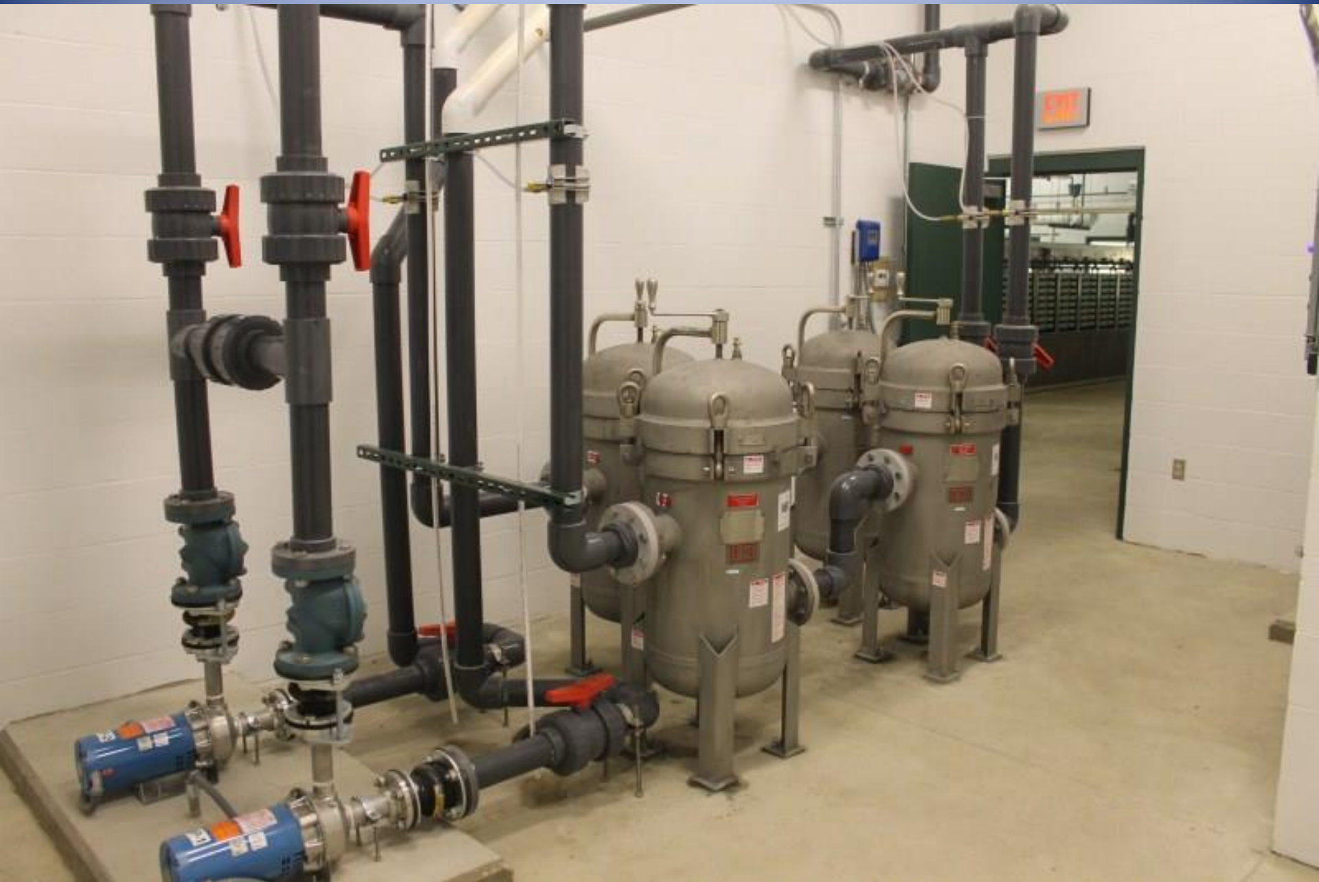
Stainless Steel Sediment Bag Filters and Booster Pumps – Incubation Water system
