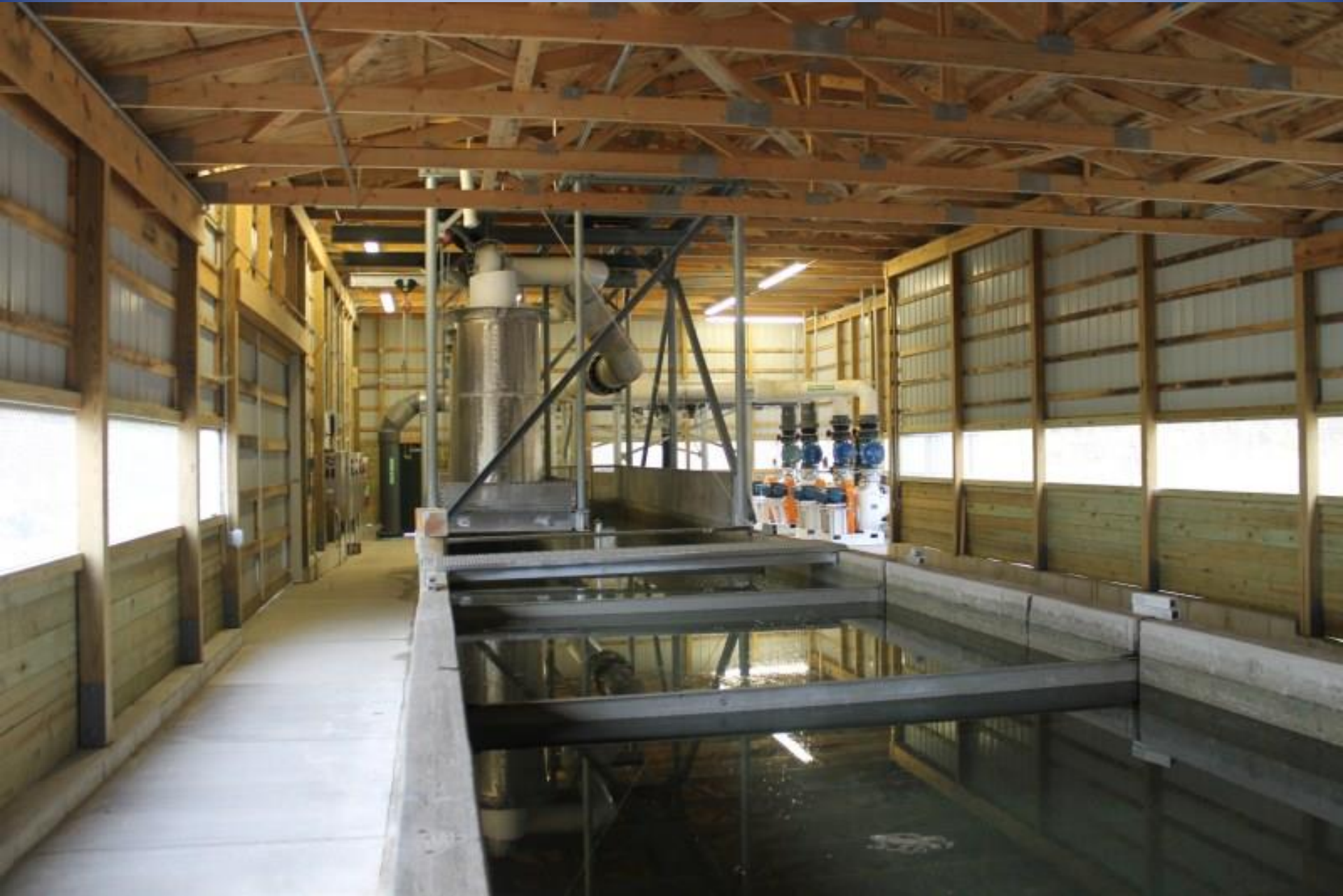
Spring Water Pumps and Aeration /Degassing Columns in Raceway Enclosure
