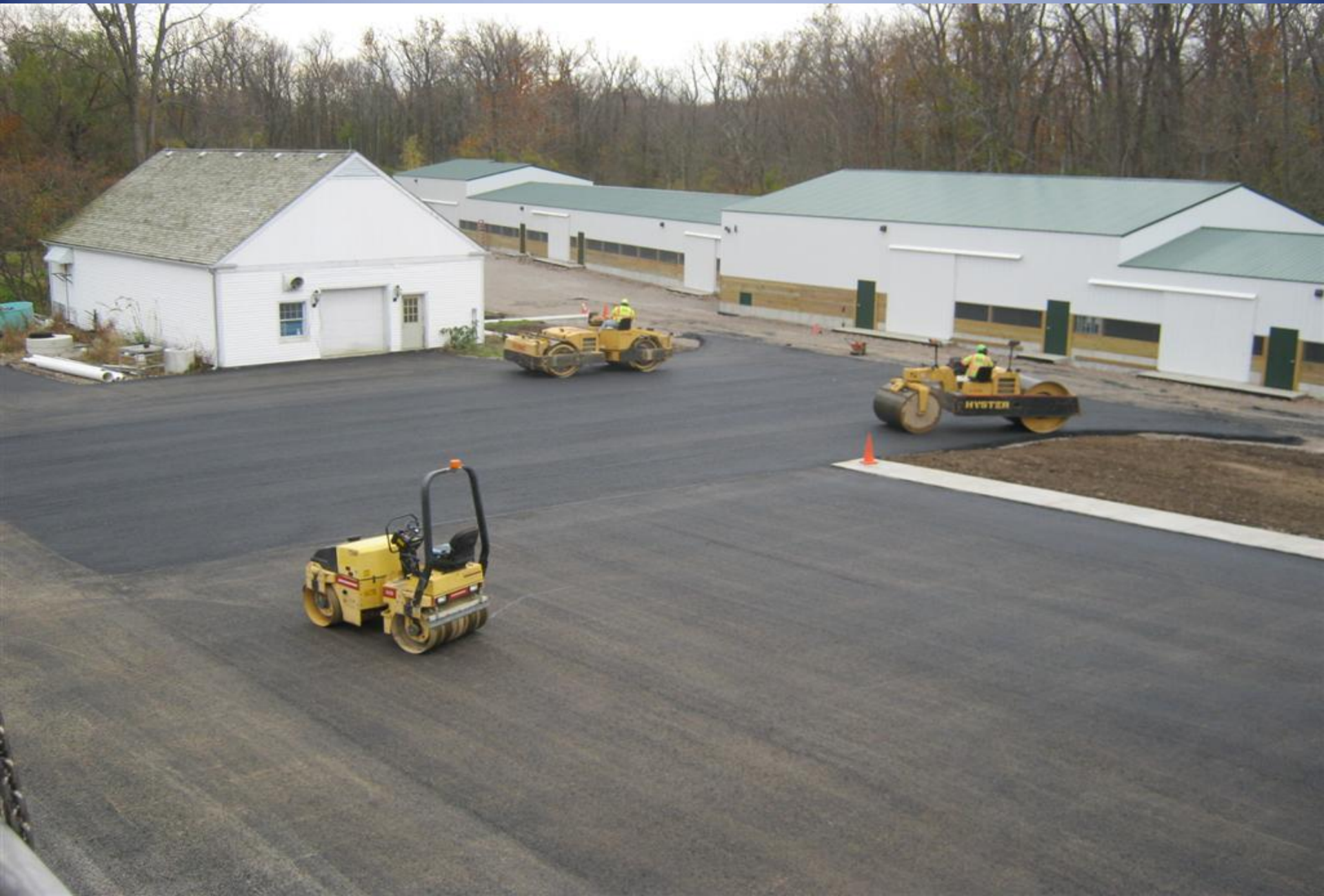
Old Production Building (left) & New Raceway Covers with Rolling Access Doors
