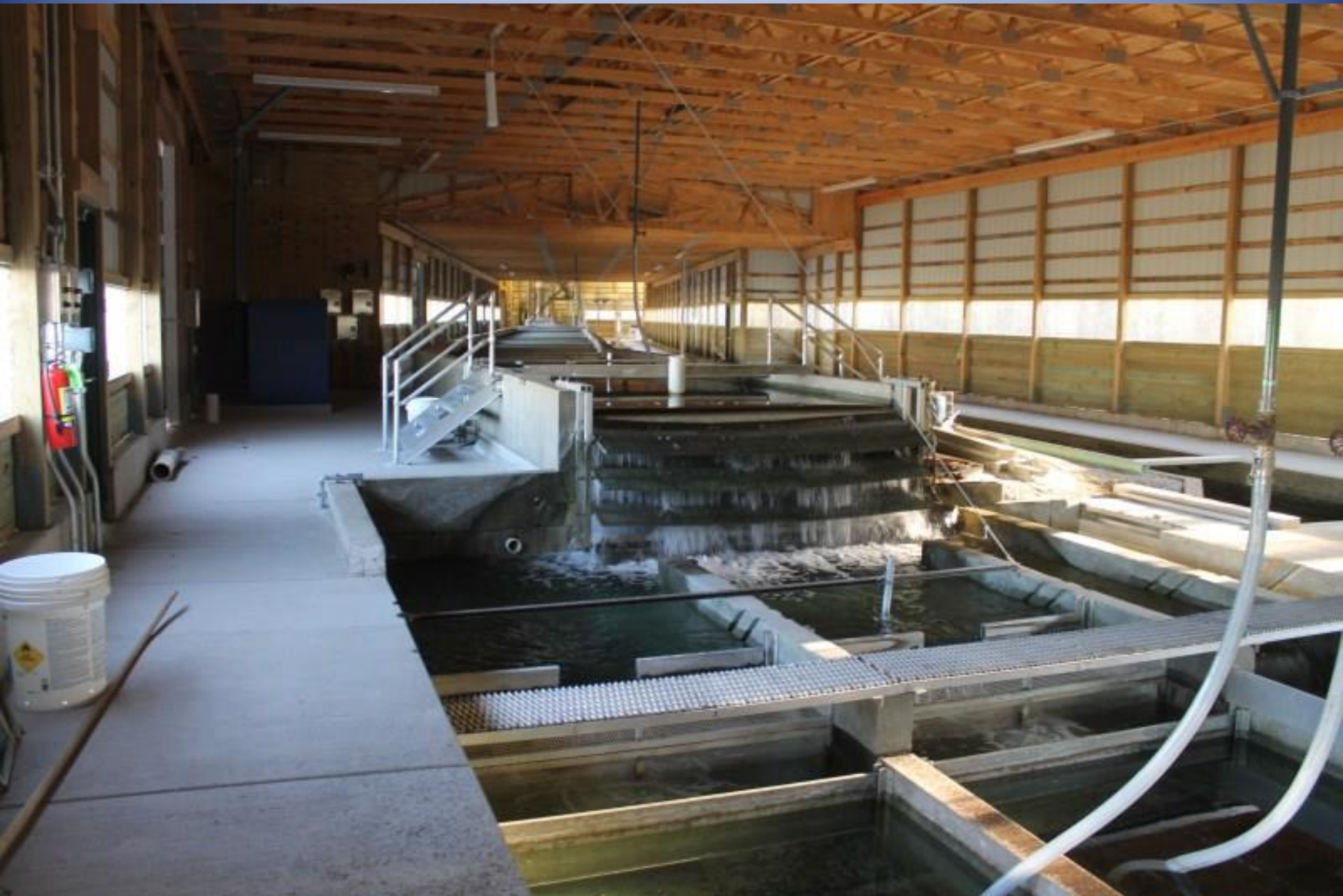
Raceway Enclosure with New VFD Operated Air Blowers and Aeration Diffusers
