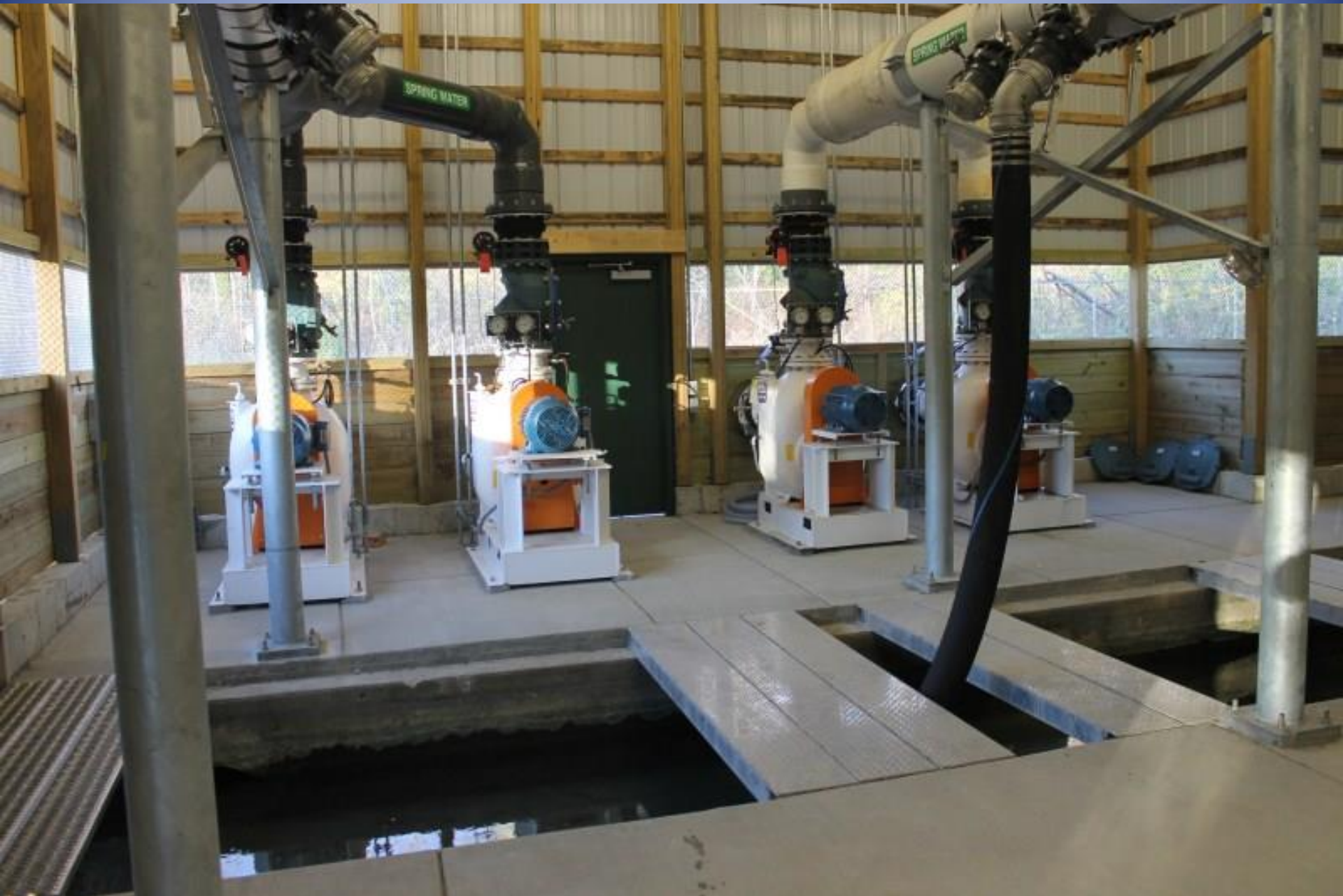
PLC Controlled Variable Speed Spring Water Pumps, 2 for Raceways and 2 for Production Building
