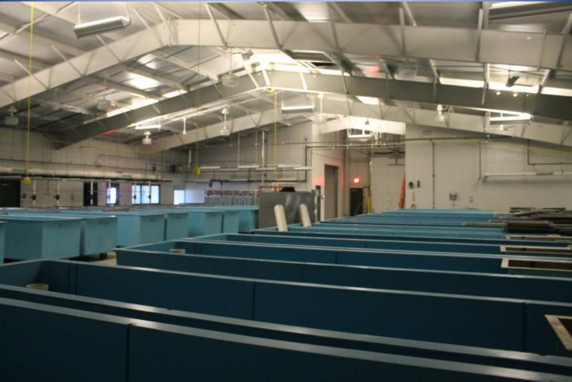
Inverted High Efficiency Fluorescent Lighting –zoned for low level fish rearing
