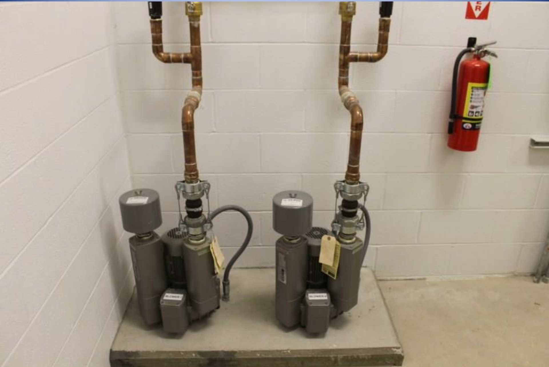
Duplex Low Pressure Air blowers – Production Building LP Air System
