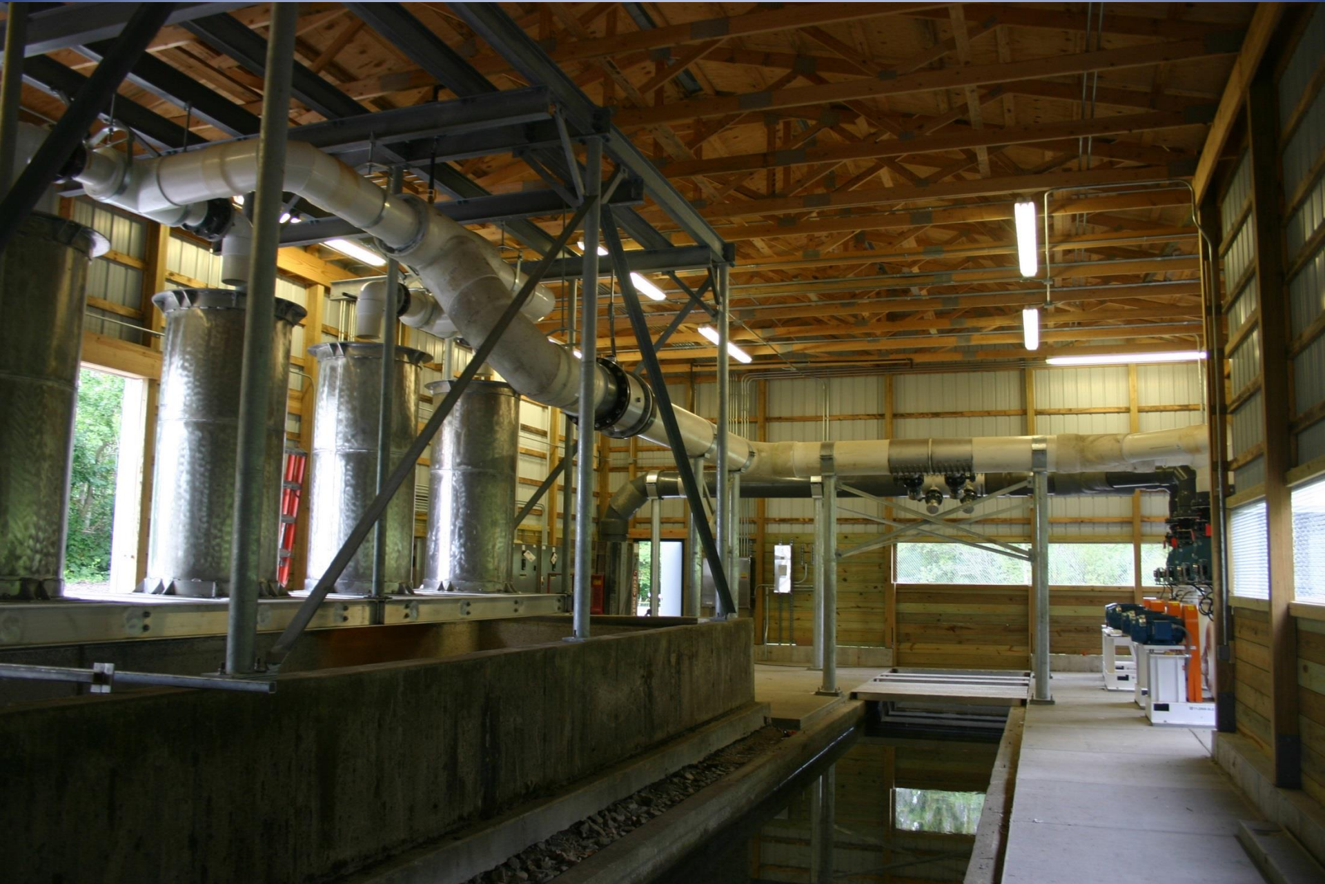
Raceway Structure – four 20 hp pumps on the right & four degassing columns on the left.
