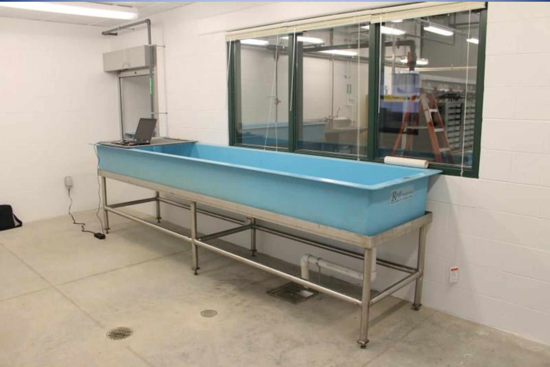
Biosecure Egg Disinfection Room – Chemical Drains to Concrete Holding Vault
