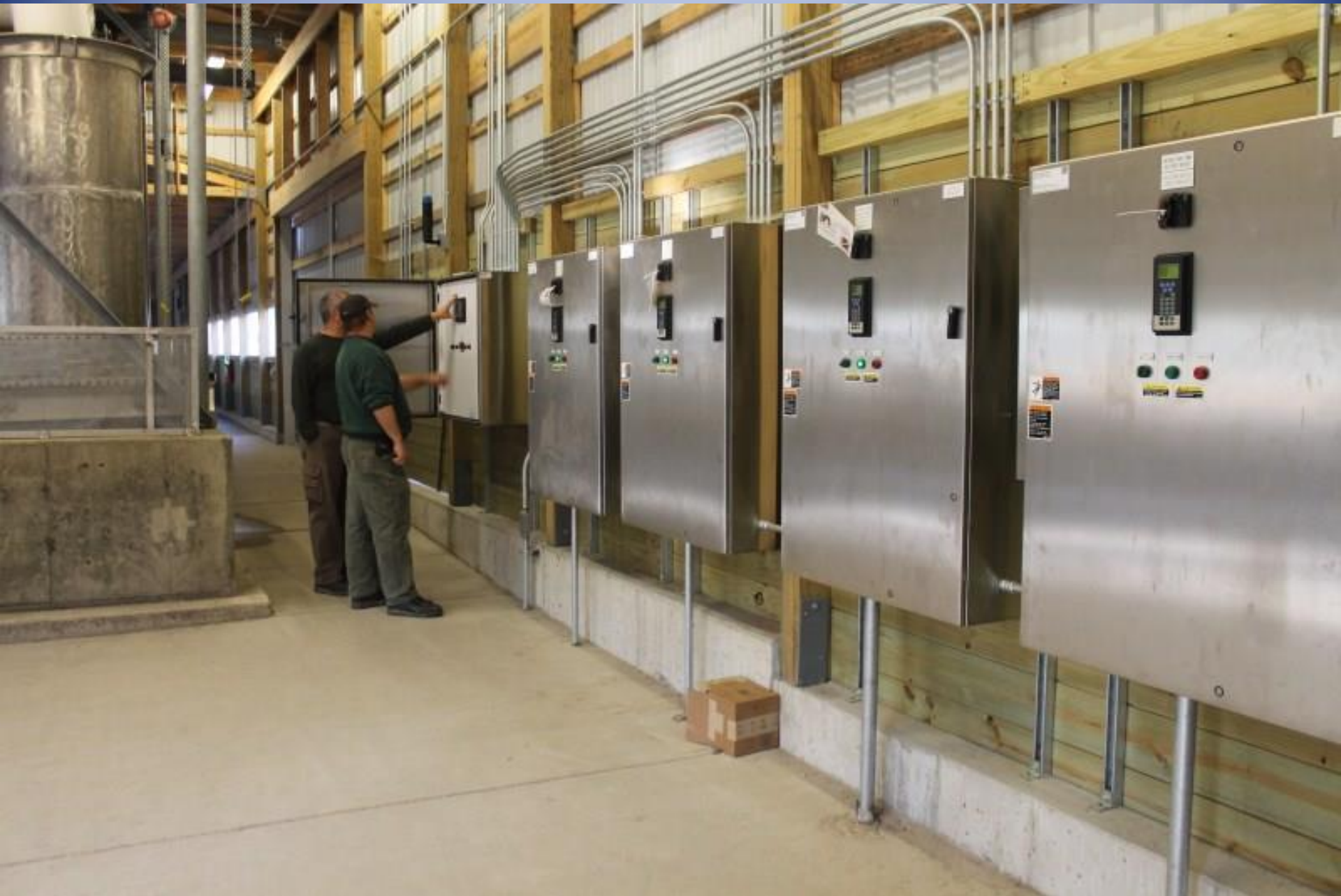
Variable Frequency Drive (VFD) Spring Water Pump Controllers
