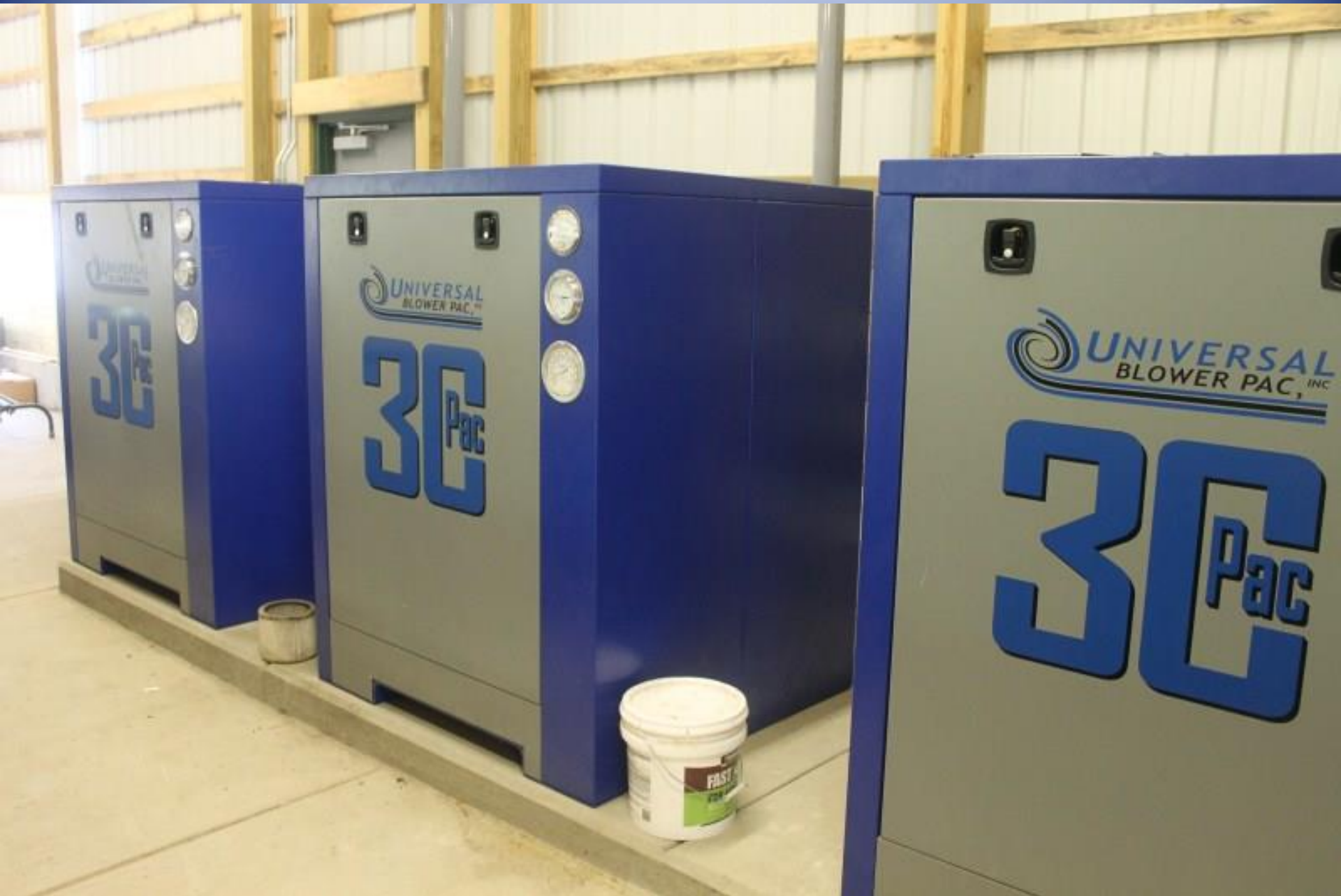
VFD Controlled Positive Displacement Air Blowers in Sound Enclosures-Raceway Aeration System
