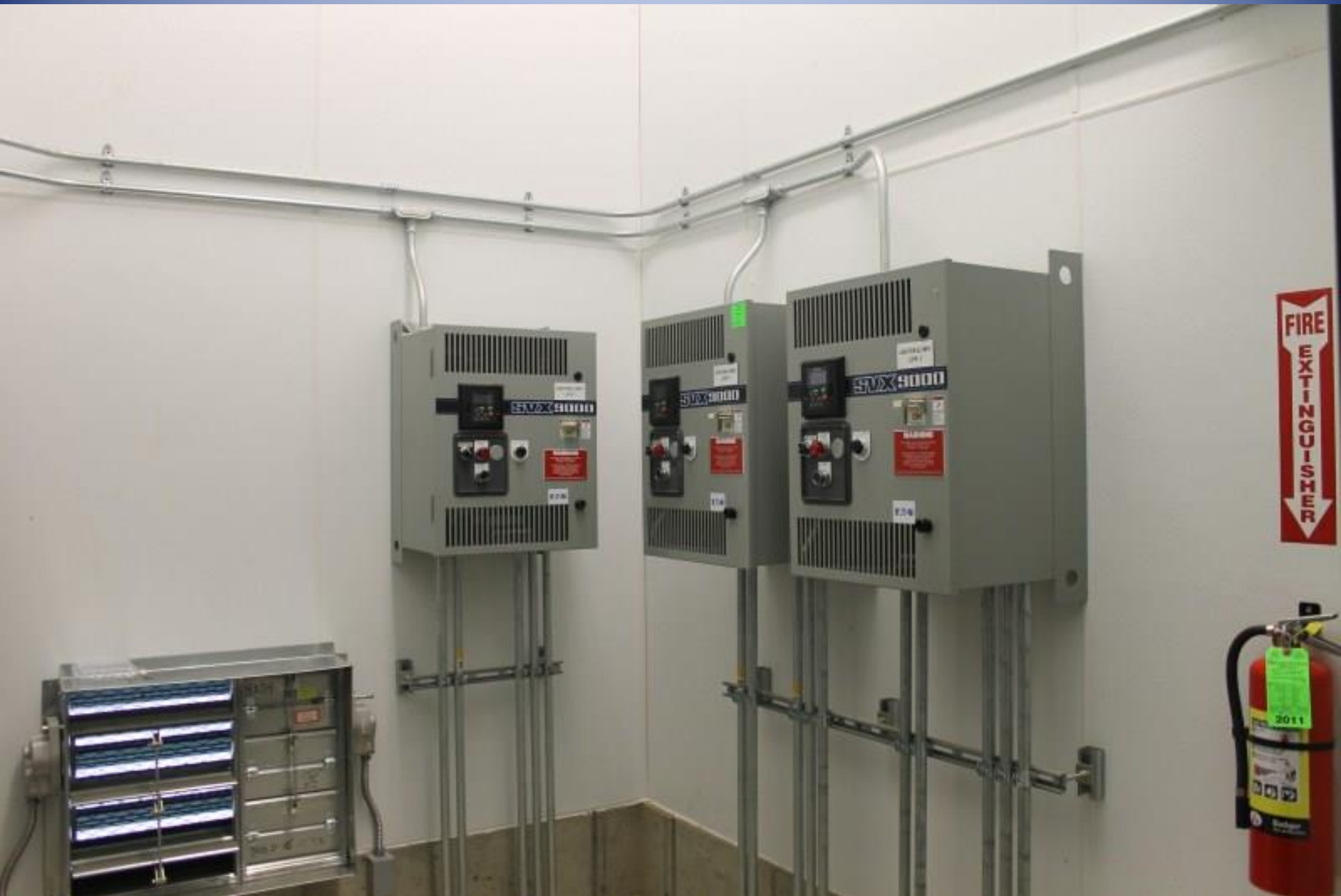
Low Pressure Air Blower Variable Frequency Drive Controllers-Air Production Output Meets Aeration Needs
