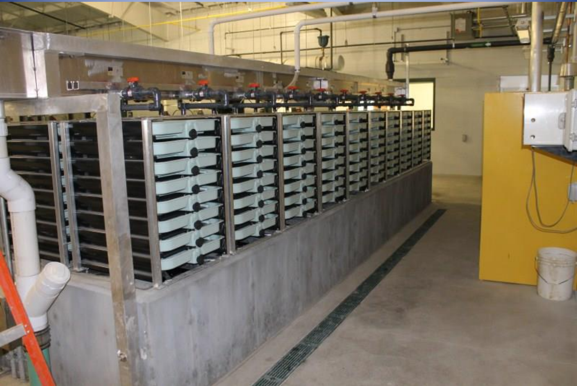
Vertical flow Egg Incubators with Bag Filtered Water Supply & Chemical Metering Systems
