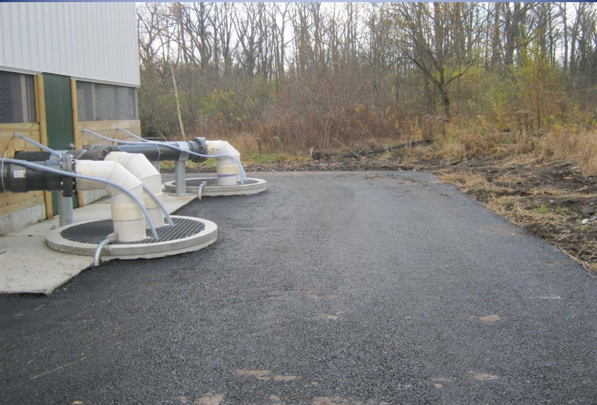
New Water Spring Water System Pump Intake Manholes
