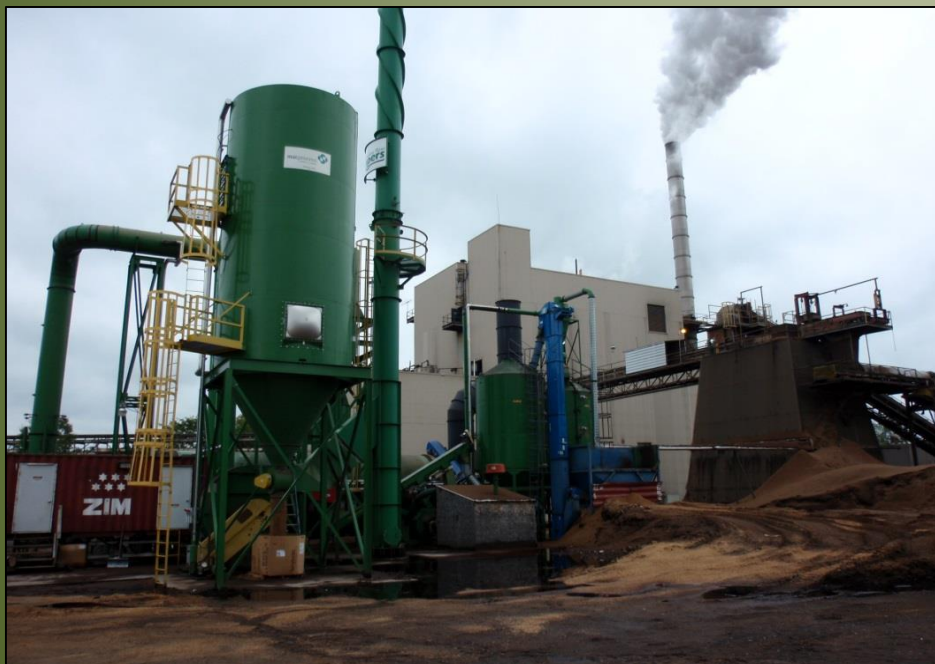
Paper mill power plant
