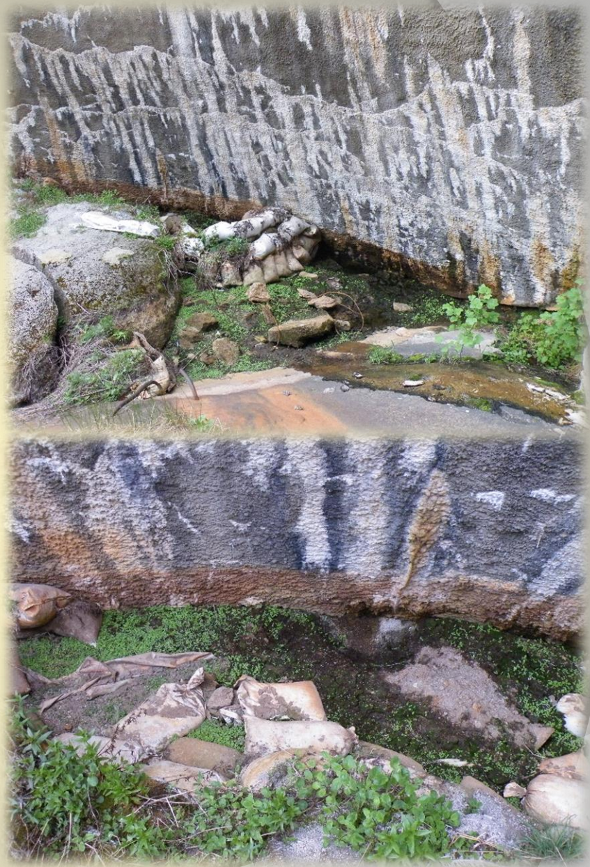
Bay 4 foundation seepage has essentially been eliminated. Seepage through the dam structure has been eliminated. Preconstruction pictures are on the left.
