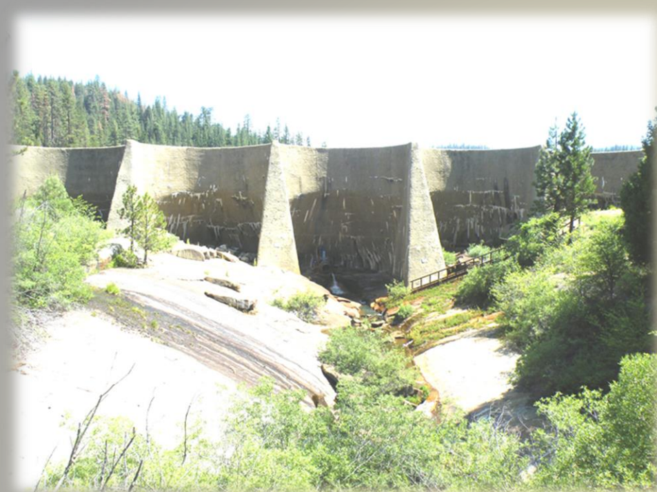
Downstream face 2015. Significantly increased seepage on the West side (right side of picture) has encouraged plant growth.
