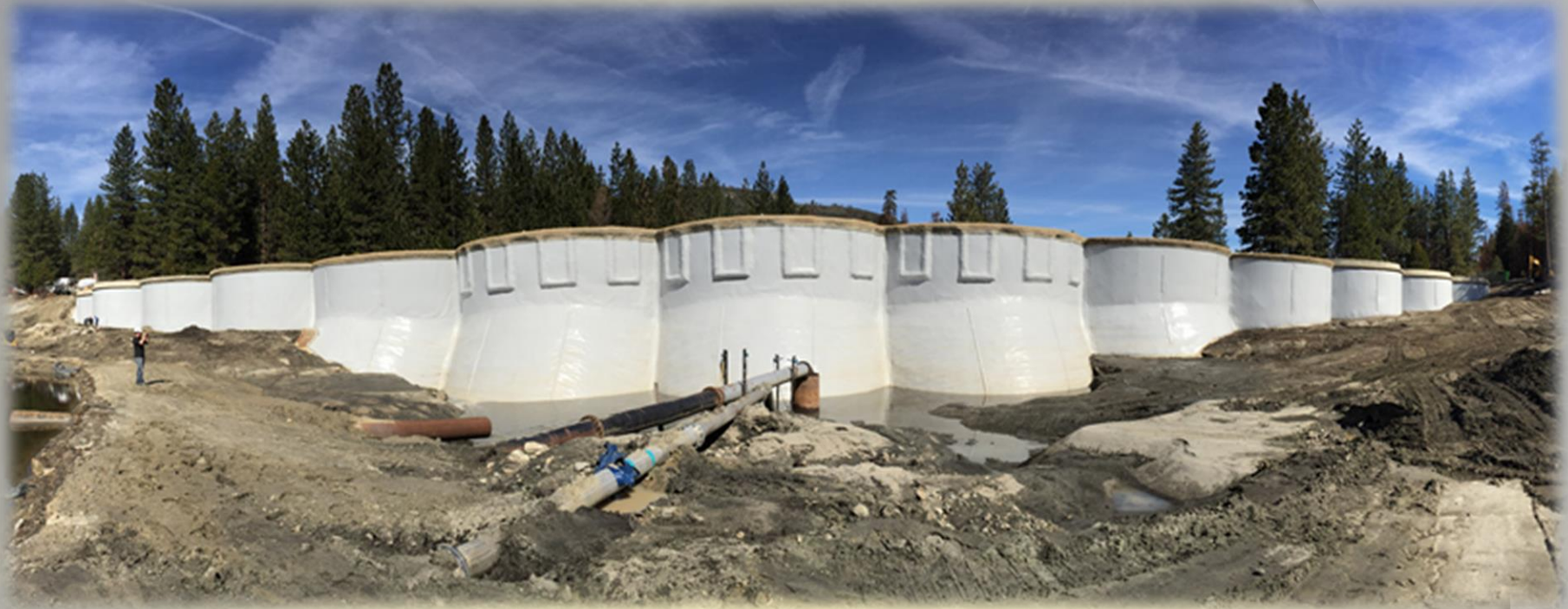
Panoramic view of Hume Lake Dam after the completion of foundation grouting and membrane installation – March 2016
