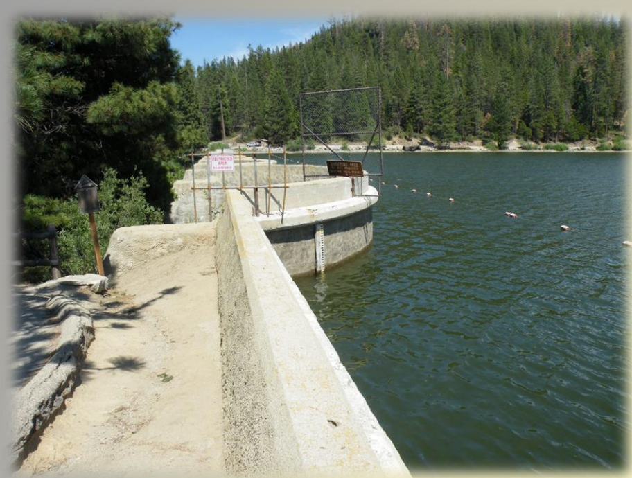
Upstream side of Hume Lake Dam 2015. Reservoir at 4.5 feet below sill with .25 to .5 cfs seepage in Bay 4
