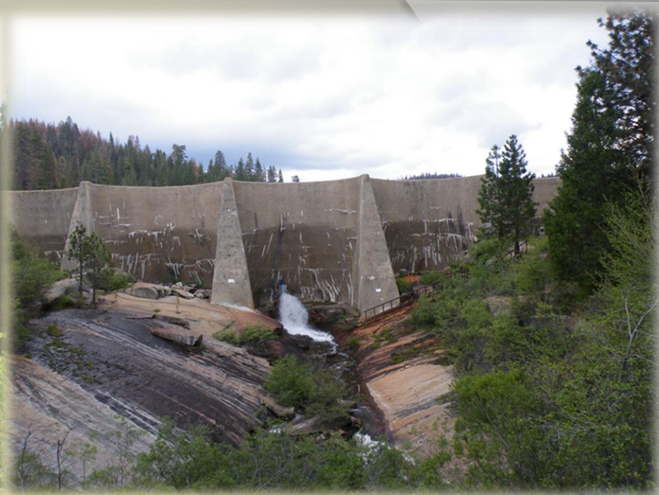
Post Construction 2016 - seepage through the entire dam has been in effect eliminated. Seepage in the West side dam foundation has been significantly reduced or eliminated.
