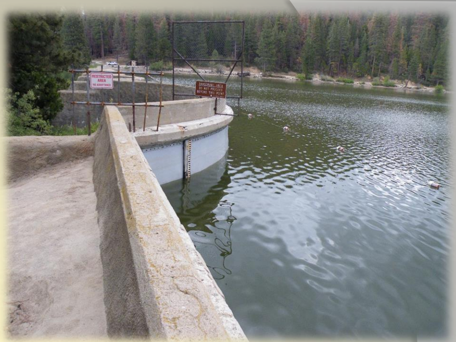
Upstream side of Hume Lake Dam 2016. Reservoir at 4 feet below sill with 0 cfs seepage in Bay 4.
