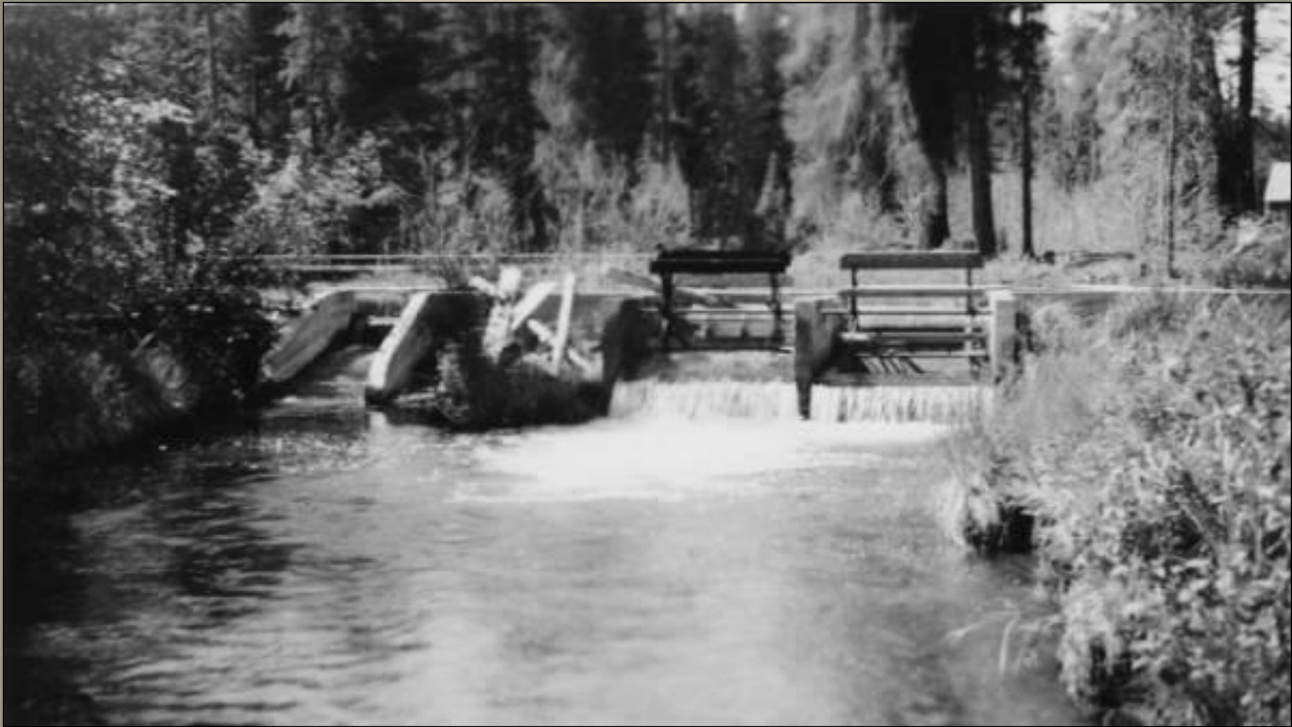
Rotating screens and spillway in power dam at the Suttle Lake outlet, 22 June 1942.
