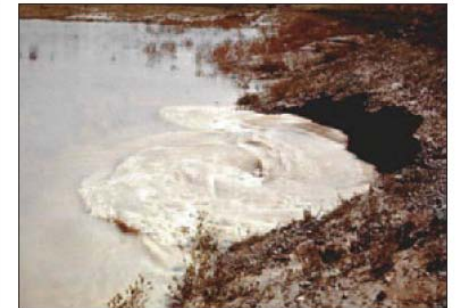
Figure 6—Whirlpool action is an indication of advanced piping.
