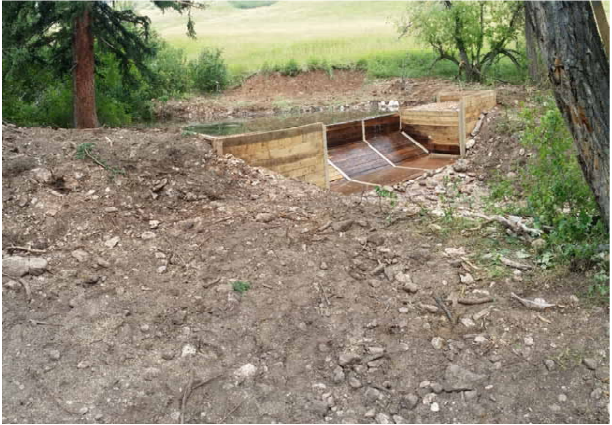
West Pass Creek Fish Barrier – Yellowstone Cutthroat Rehabilitation Project-upstream barrier constructed in 2018.
