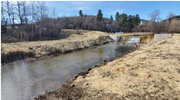
Fish barrier to limit brook trout passage in order to restore the yellowstone cutthroat population.
