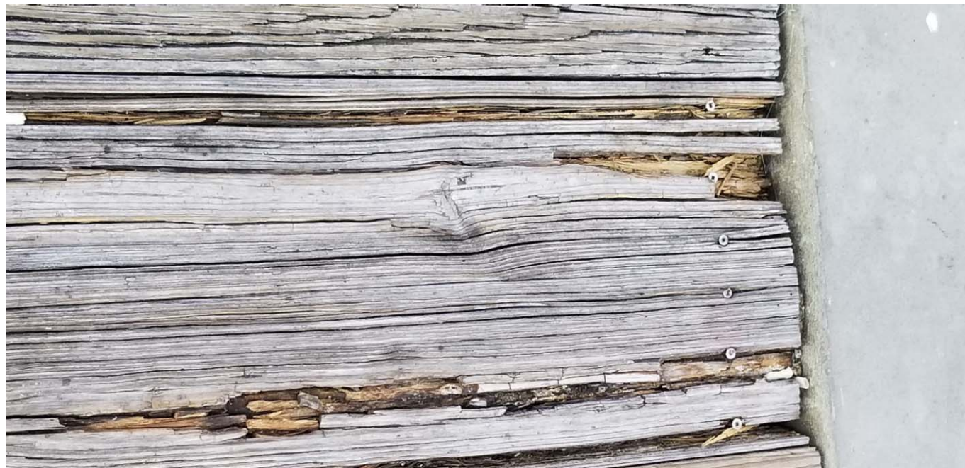
EXISTING DECK DELAMINATION
