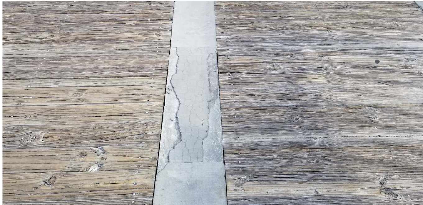
EXISTING CONCRETE DELAMINATION
