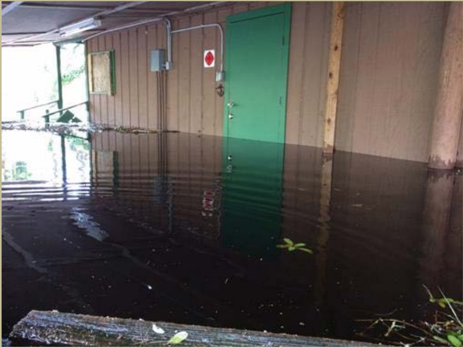
Flooding at cabin caused by Hurricane Irma
