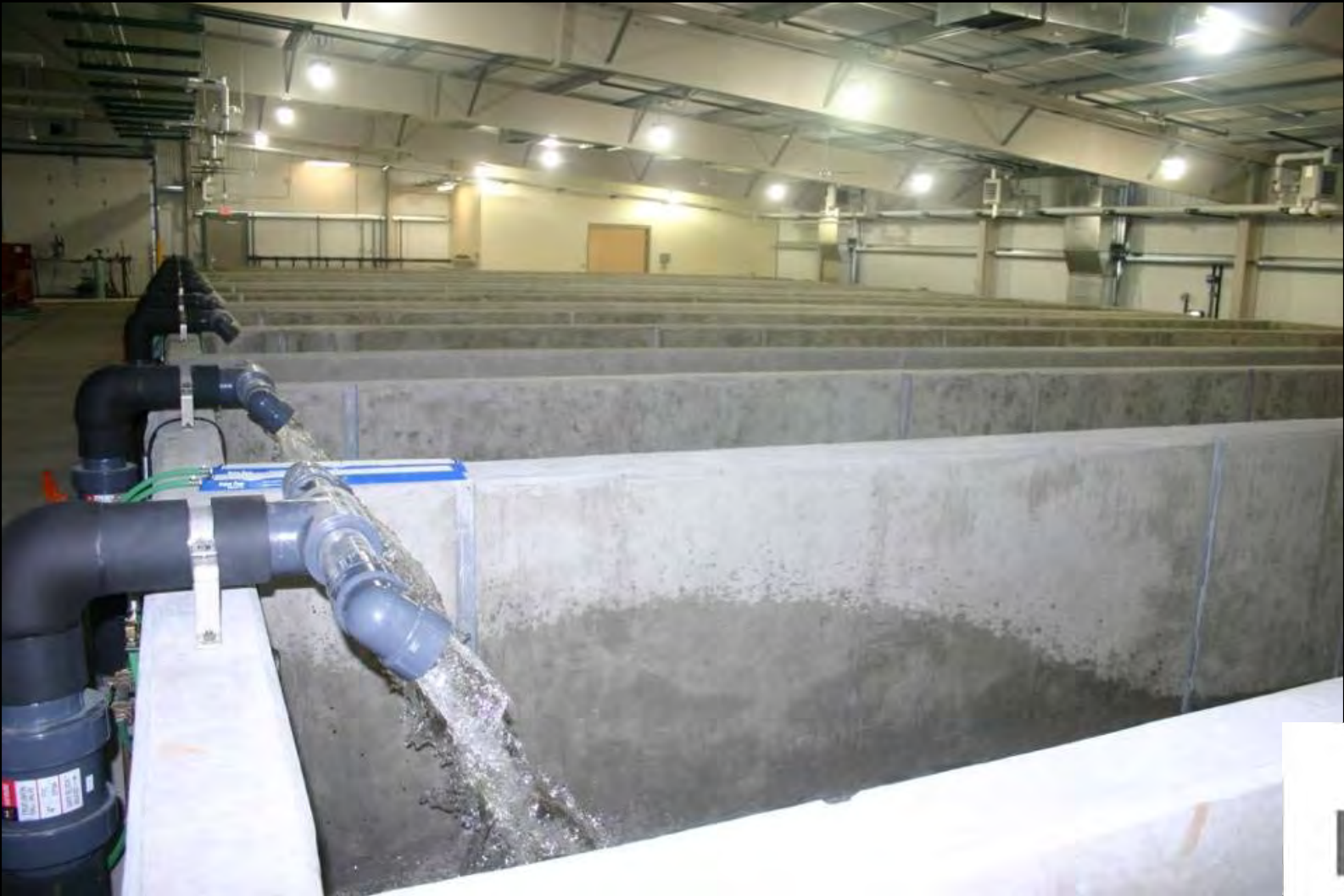
50ft x 6ft Broodstock Raceways in Biosecure Bldg.
